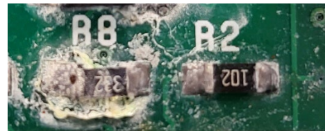
Figure 3-5. Corrosion on Circuit Board
